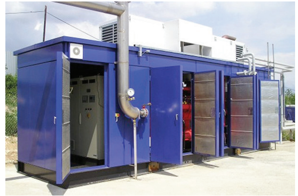
CHP unit Úholičky, CZ, 520 kW Waukesha, prod.capacity 3.500 MWh/year.
